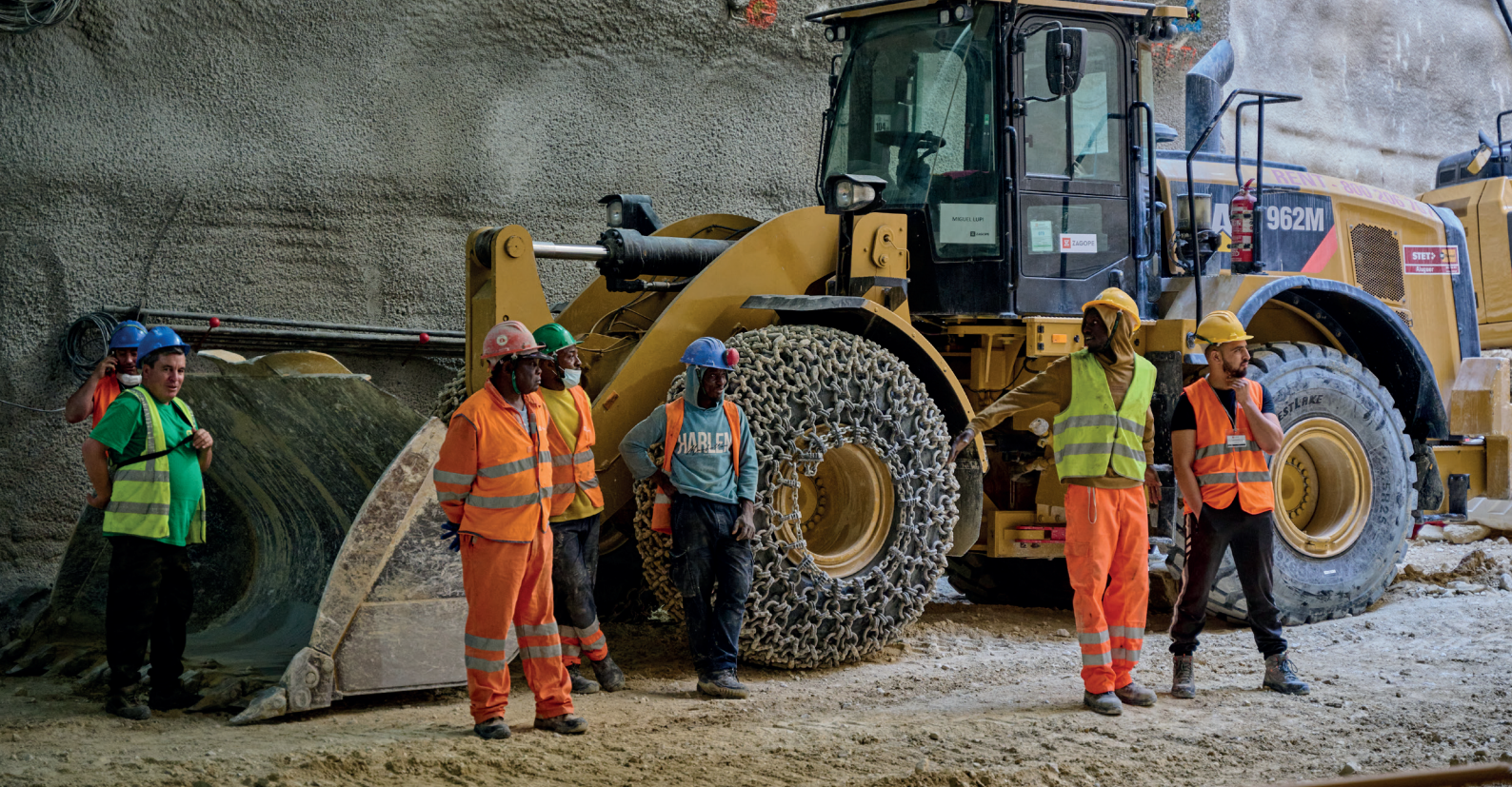
Workers stand in front of large machinery as they wait for the wall to be breached at the future Estrela underground station on May 28, 2022 in Lisbon, Portugal. © Horacio Villalobos/Corbis via Getty Images
